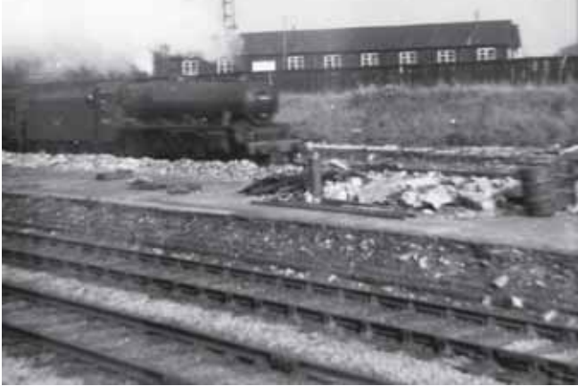
Photo taken during the demolition of Farington Station in 1960. Courtesy of Dave Ellithorn. Jubilee Class No. 45663 'Jervis'
